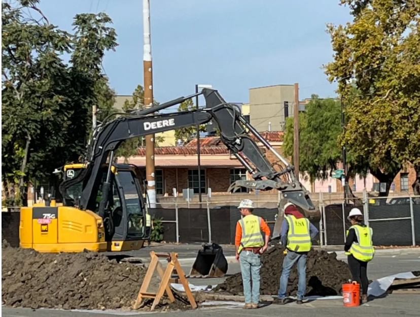
Construction crew watches as an excavator move dirt and rubble on a downtown San Jose parking lot near the former site of the now-rescued Stephen's Meat Products (Dancing Pig) sign at 81 S. Montgomery St. (George Avalos/Bay Area News Group)
